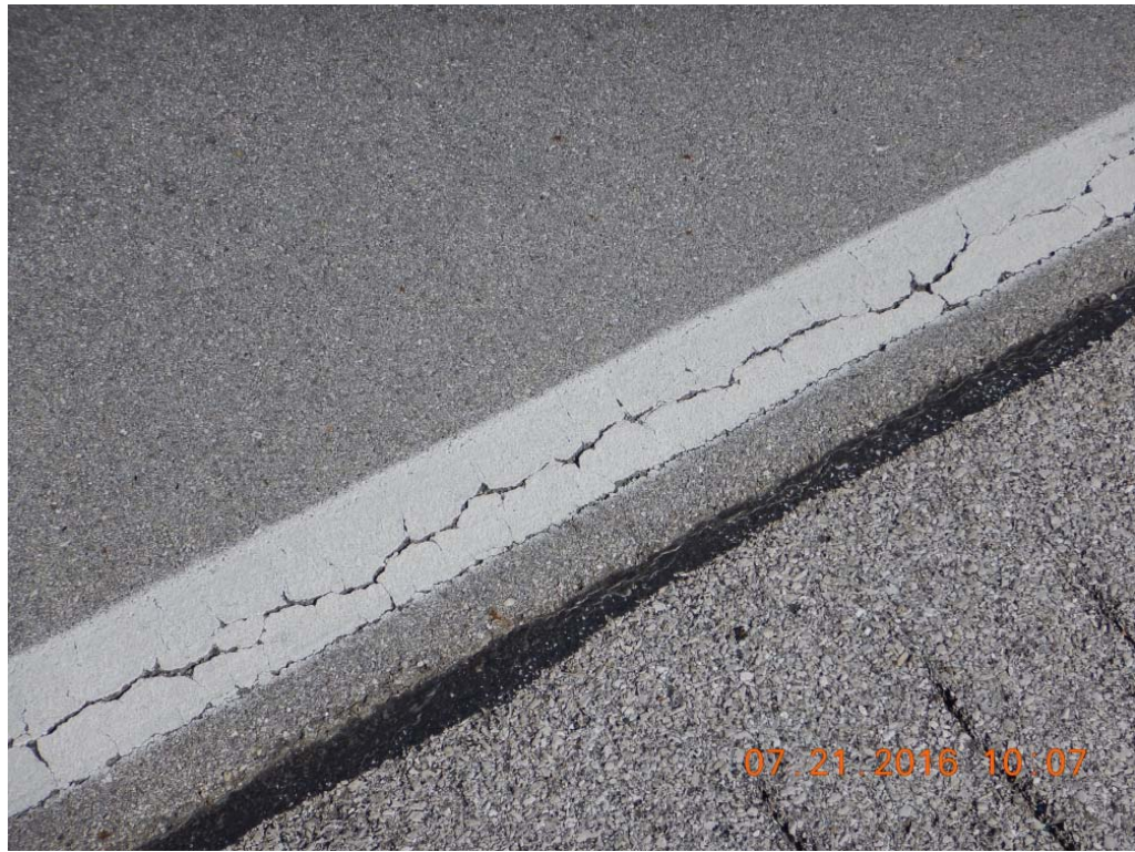
Figure 7.5: Pulaski County, Edge Cracking, Thinlay
