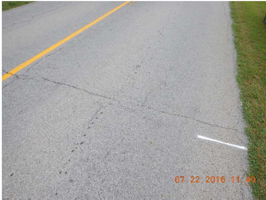
Figure 7.3: Green County, Longitudinal/Transverse Cracking, Thinlay
