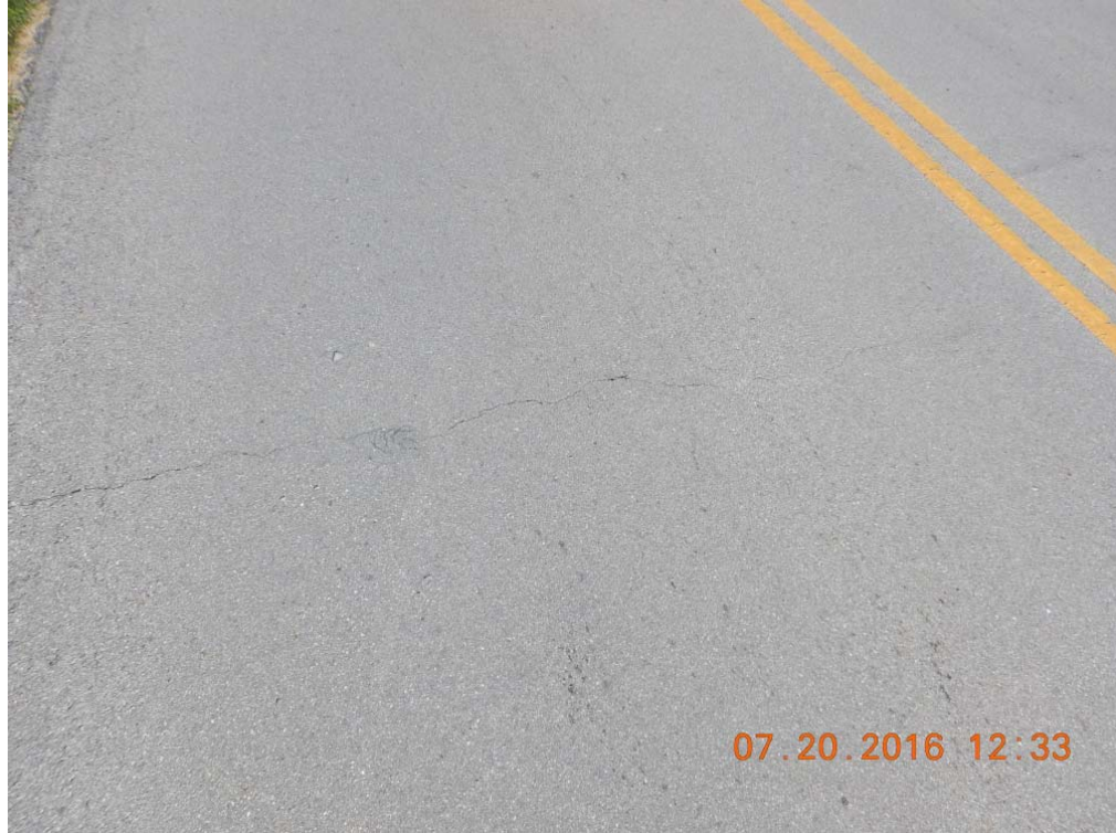
Figure 7.6: Laurel County, Transverse Cracking, Microsurfacing
