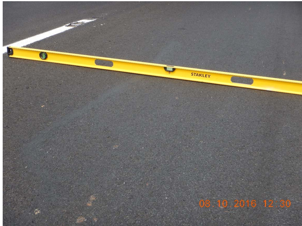
Figure 7.15: Warren-Allen County, Rutting, Fresh Microsurfacing
