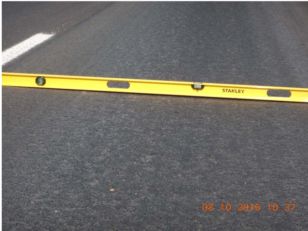
Figure 7.14: Warren-Allen County, Rutting, Fresh Microsurfacing
