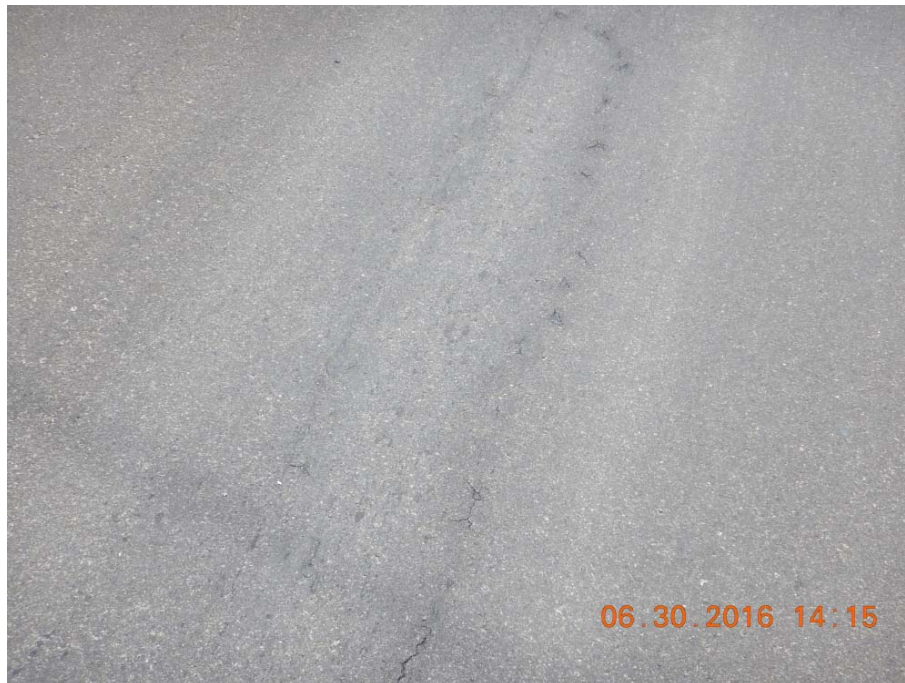
Figure 7.2: Morgan County, Bleeding Distress, Brand New Surface
