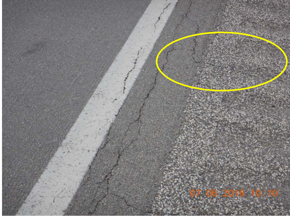
Figure 7.4: Greenup County, Reflective Crack/Edge Cracking, Microsurfacing
