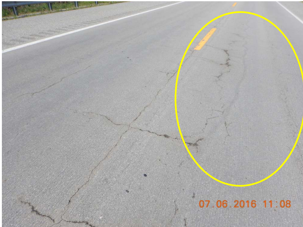
Figure 7.8: Greenup County, Alligator Cracking, Microsurfacing
